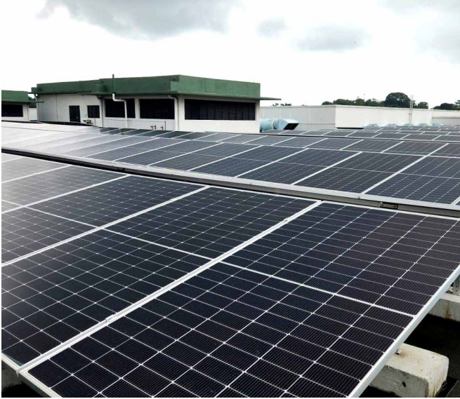
Solar panels installed at the SIA Supplies Centre
